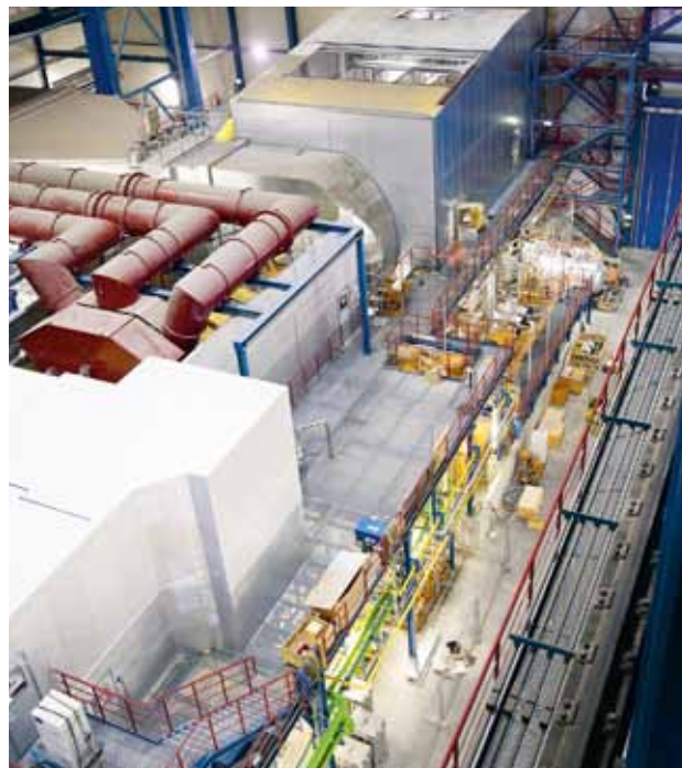
^ The combined cycle power plant boasts an efficiency of over 60 percent. The gas turbine, the generator and the steam turbine are mounted together on a single shaft.
