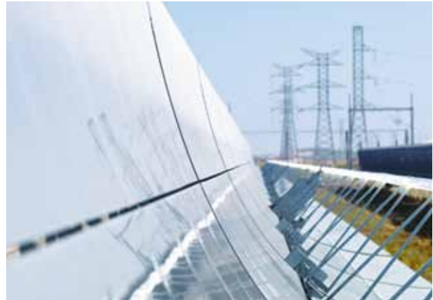
^ Giant parabolic mirrors in the Lebrija solar power plant collect the sun's energy and use it to generate electricity for up to 50,000 households.
