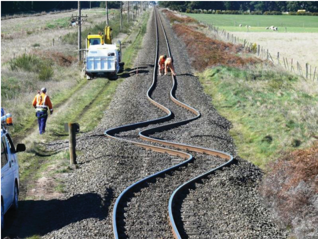
Figure 3.4 A New Zealand Railbed after an Earthquake
