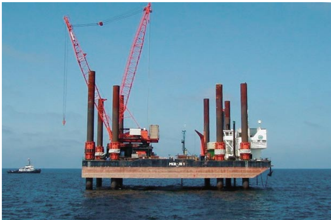
Figure A12-2: Drilling and conic penetration test with a platform from Mohiba.
