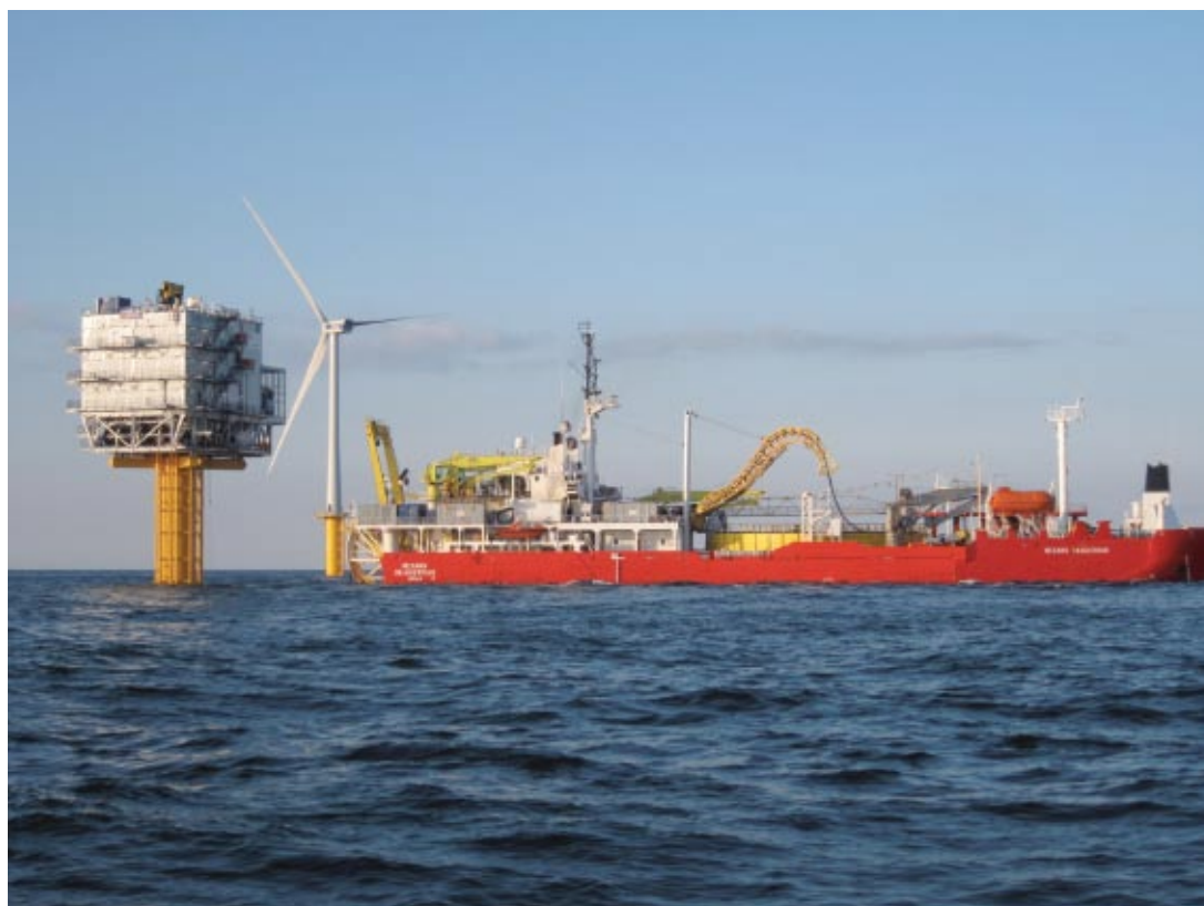
Figure A9-2: The Skagerrak pull the export cable to the OHVS at Belwind. (Courtesy of the Belwind organization)
