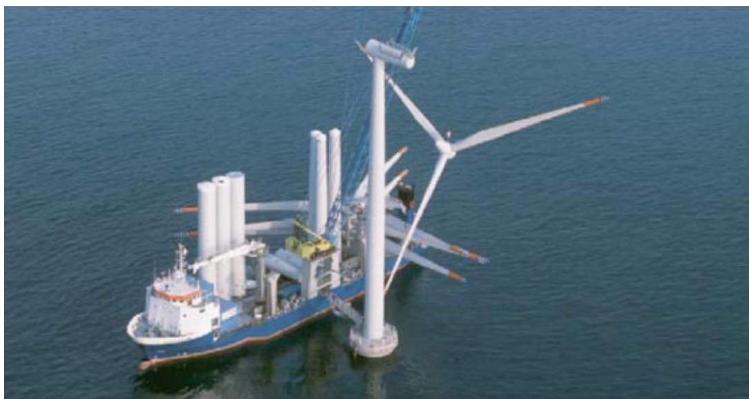
Figure A2-2: Installing Siemens turbine with the MS Ocean Ady. (Source Siemens Wind power)
