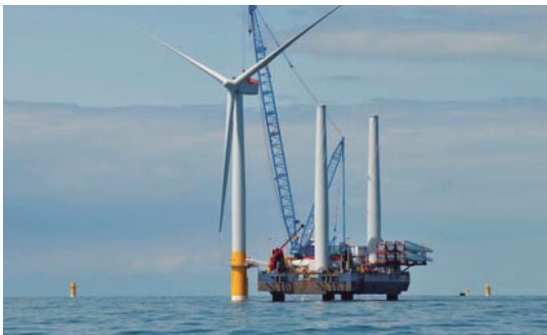
Figure A10-2: First turbine installed at the Greater Gabbard offshore wind farm. (Courtesy of SSE and RWE npower renewables)
